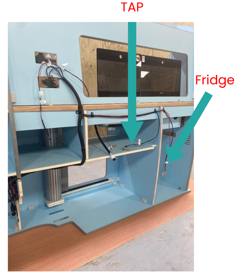
Using the cut outs in the furniture, run the fridge and tap cables into place and p clip into position
