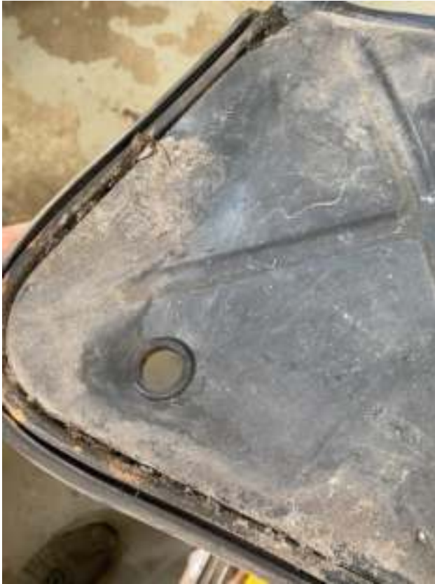
Cut and fit a rubber grommet to the cover above the battery
