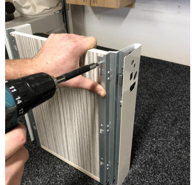
Fit the drawer base using 16mm screws, ensure the base is flush to avoid gaps
