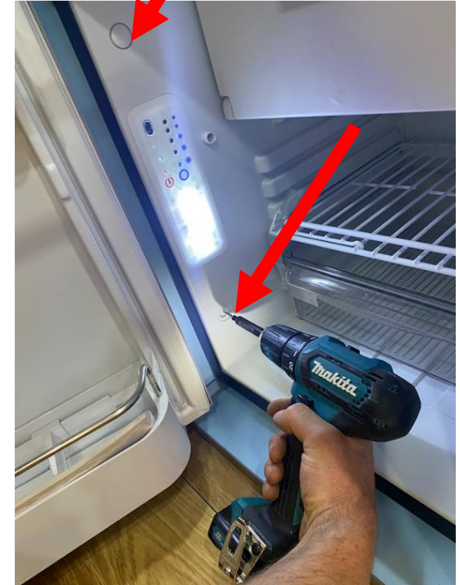
Remove the fridge fixing point caps, screw through into the aperture, use 30mm screws, be mindful not to screw through the ply
