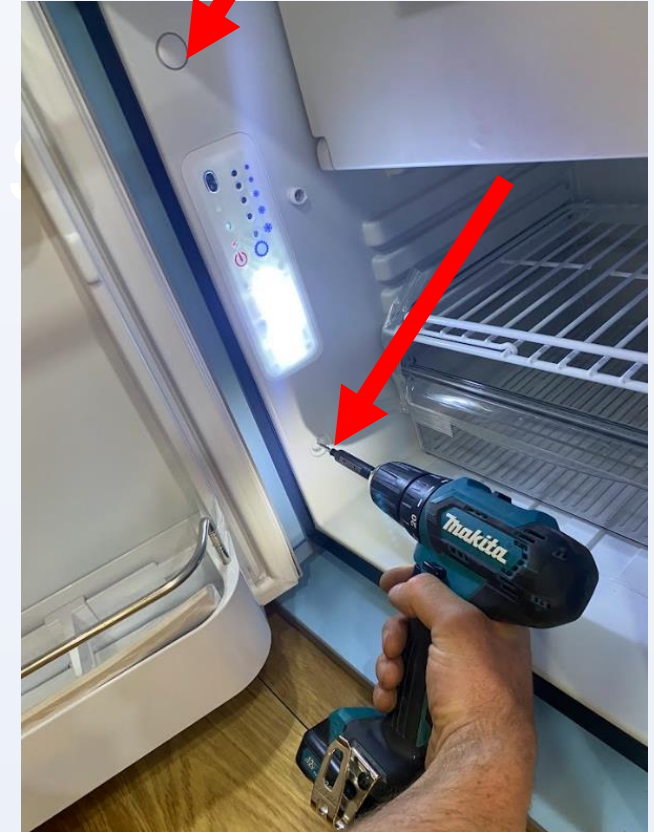
Remove the fridge fixing point caps, screw though into the aperture, use 30mm screws, be mindful not to screw through the ply
